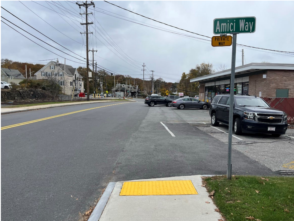
Figure 46. Missing Sidewalk on Railroad from Amici Way Through the Laundry Mat Parking Lot. (Tony Collins).
