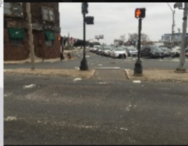
Crosswalks need repainting
