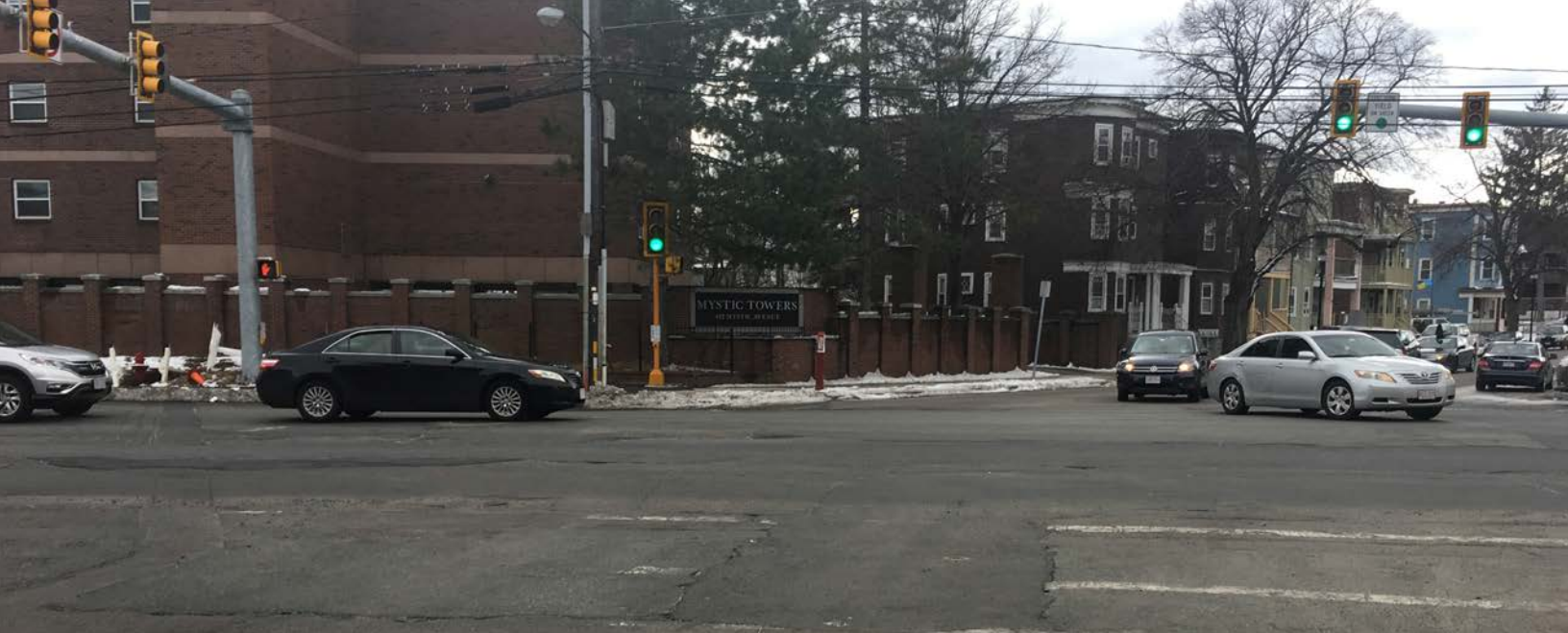
Crosswalks Along Busy Mystic Ave, Right In Front Of The High Density Housing Complex Mystic Towers, Are Severely Degraded. Photo: Liza Burkin.
