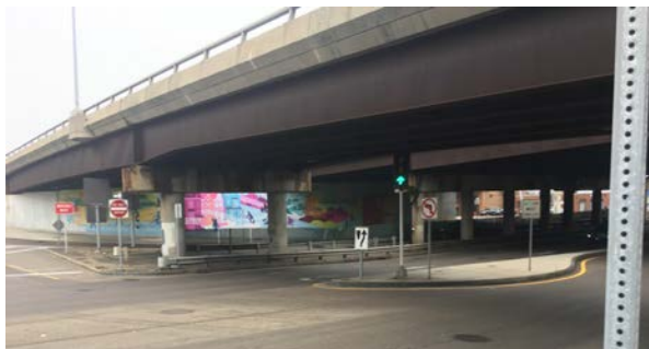
I-93 Underpasses Along The Mystic River Create An Uncomfortable Pedestrian Environment. Photo: Liza Burkin.
