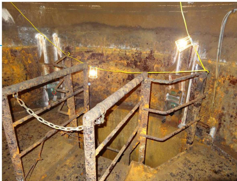
Figure 4 Image of monopile interior without proper corrosion protection (from Lichtenstein 2015)
