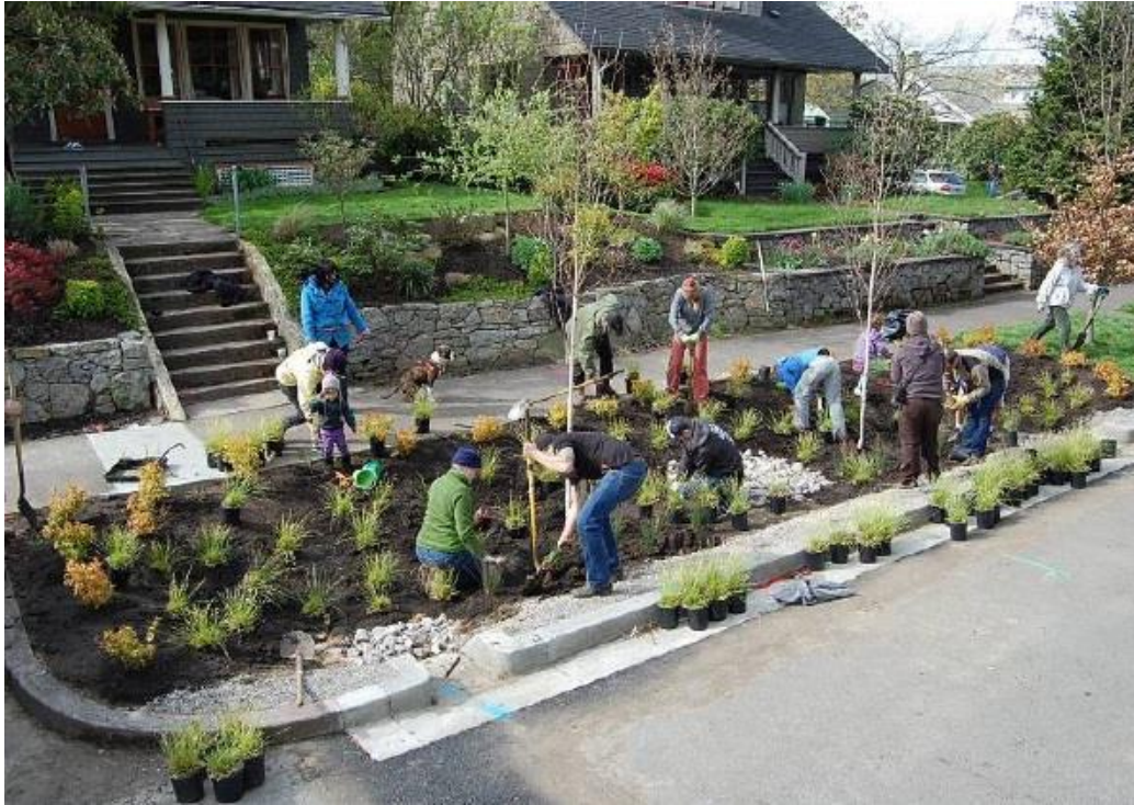
Figure 4: Portland, OR. Installation day with Portland Green Streets Program. (Source: Museum of the City, 2017.)
