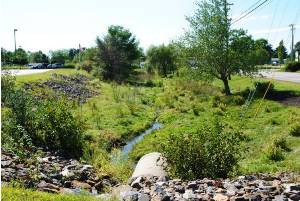
Figure 8: Long Creek Watershed, South Portland, ME. Blanchette Brook Stream Restoration. (Source: Long Creek Watershed Management District, 2016.)
