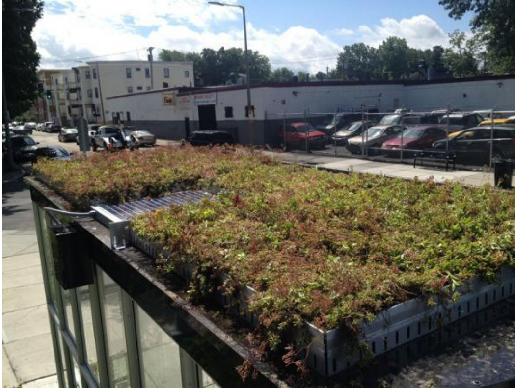
Figure 13: Bus Shelter Green Roofs, Boston, MA. A living roof on a Dorchester bus shelter. (Source: Dorchester Reporter , July 31, 2014.)
