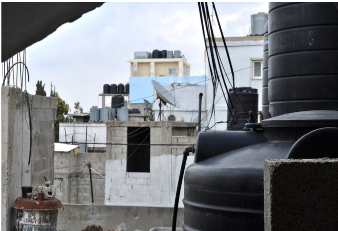
Rooftop water tanks in al Azza refugee camp
