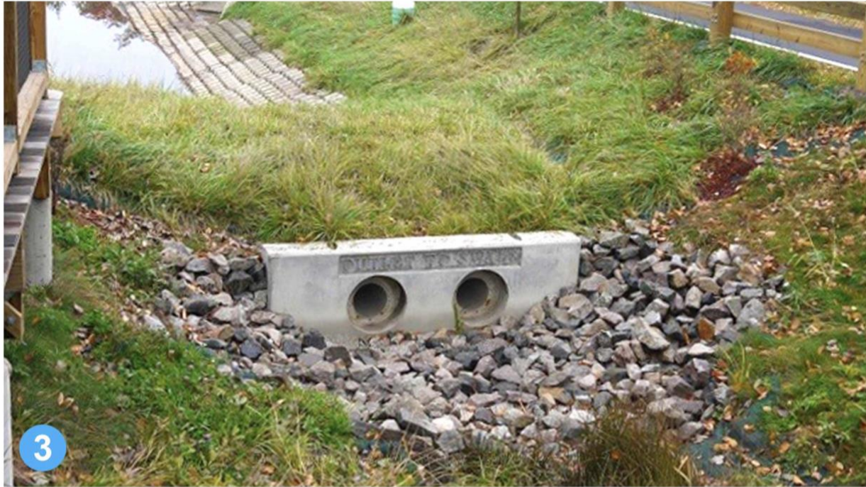
Cross berm outlet, (2) 12-inch RCP pipes leading to water quality swale (looking East)
