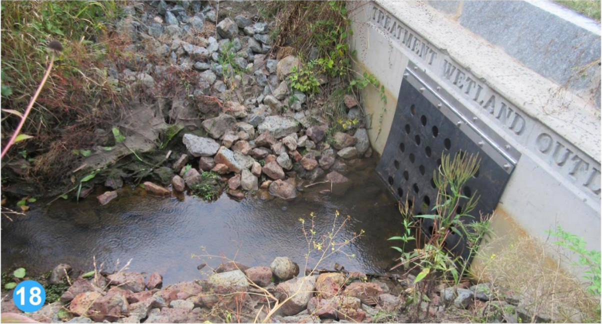
36" flexible fish flap gate at stormwater wetland outlet
