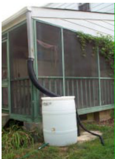
Figure 15. Example of a Rain Barrel Used to Capture Residential Rooftop Runoff
