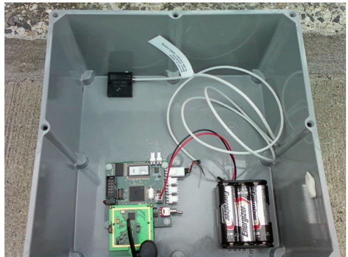
Figure 23: Inside the PVC Fitting
