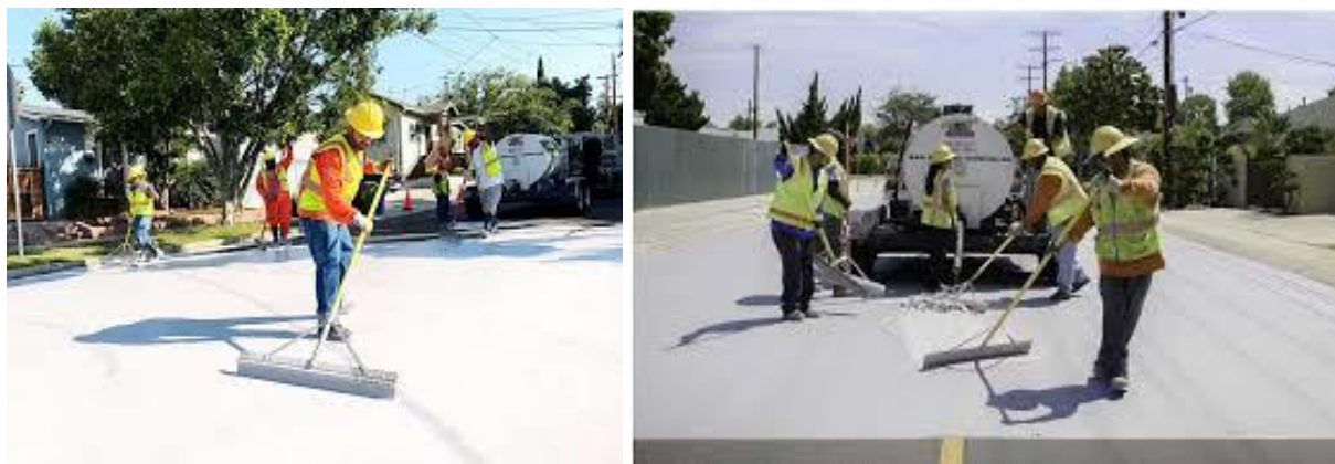
Figure 7. CoolSeal Project in Los Angeles. Photo credit: City of Los Angeles Public Works
