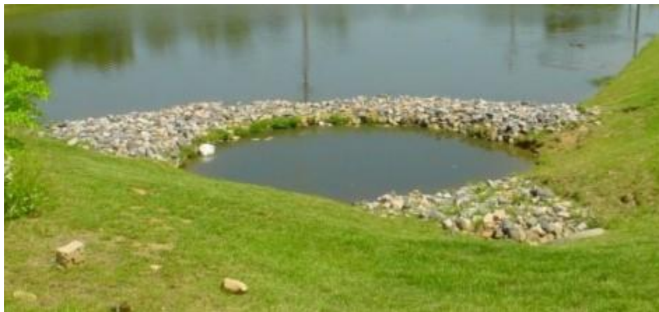
Figure 18: A sediment forebay. Source: Massachusetts Clean Water Toolkit.
