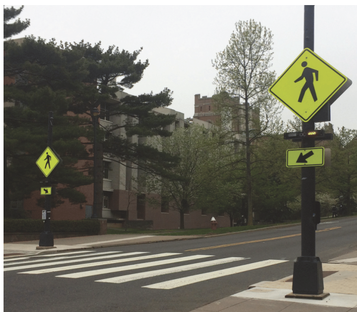
Figure 30. RPFb user activated pedestrian cross signal. Source: Federal Highway Association.
