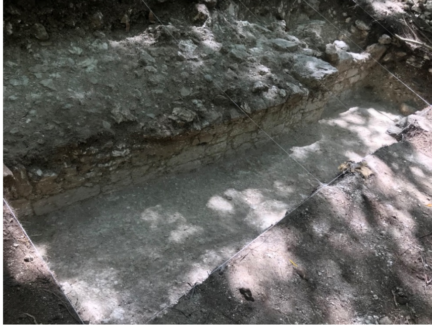
Figure 1: Structure 5, Las Abejas, Belize. This photo shows how the once vertical wall is now leaning slightly outward (see top right – the wall is not perpendicular to the leveled floor) and that the top stones in the wall were displaced to a greater degree than those at the base (why this happens is discussed in Section 2: Factors Post-Abandonment). Courtesy of the PFBAP.
