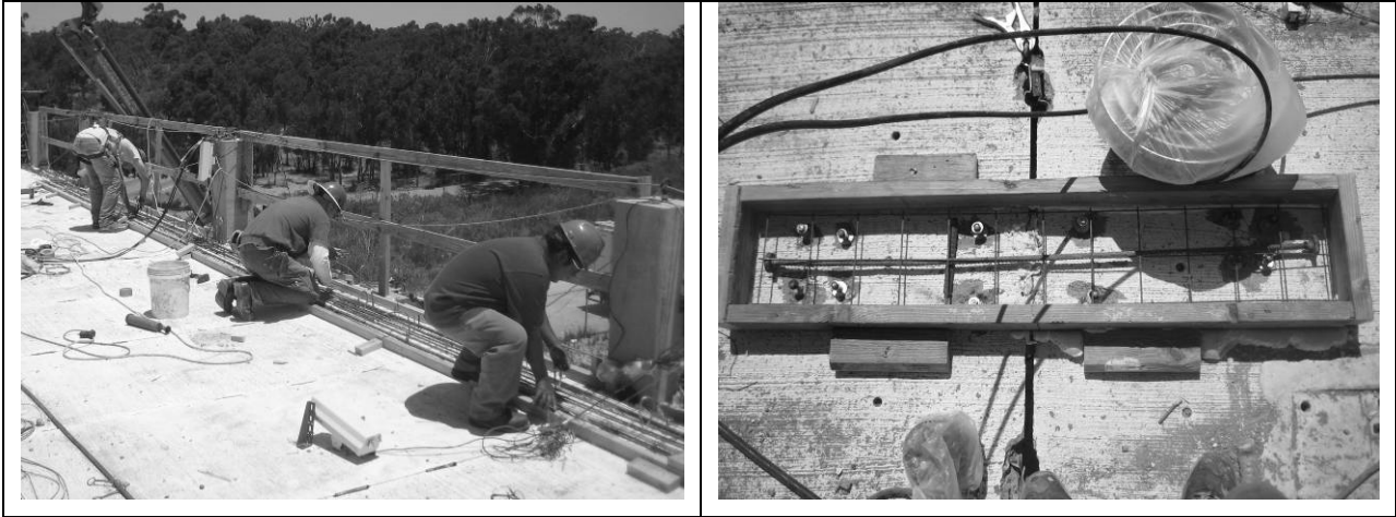
Figure 17 – Flexural chord and mid-span shear repair of third floor before test T18.
