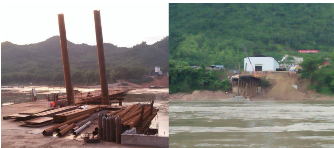
Photo8: Bridge across Mekong River by the CREC No8 near Luang Prabang (June 24 25, 2017)
