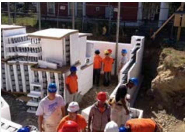
Students learning carpentry skills at Madison Park Technical Vocational High School and building a home on DNI. The project is in partnership with YouthBuild and Boston Carpenters Training Apprentice.
