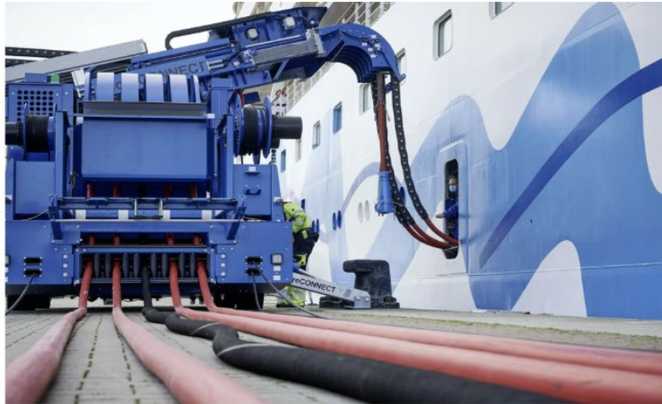
Figure 3: Shore Power Cable Management System 15
