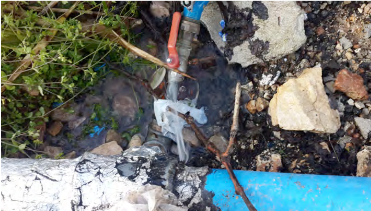
Figure 4. Leak in pipe distribution network in Al-Walaja
