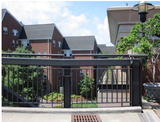
Figure 8. Deformation of top chord at its connections to Dowling Hall building
