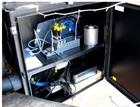
Figure 4. View inside the enclosure
