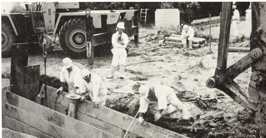
When the clean up exposes the chemicals, it can become more of a hazard than the site itself.
