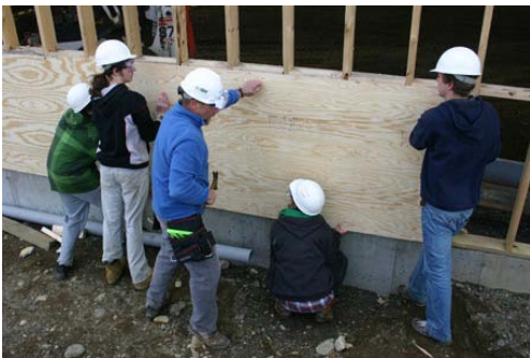
Students work along with Plant Manager to Sheath the North Wall (The Putney School, 2008, "Field House Blog")
