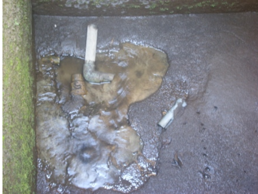
Figure 16: Accumulated sediment inside the capture tank. [55]
