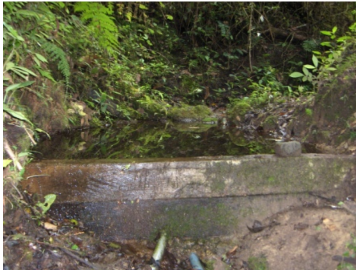
Figure 17: Capture tank for Las Tolas [55]
