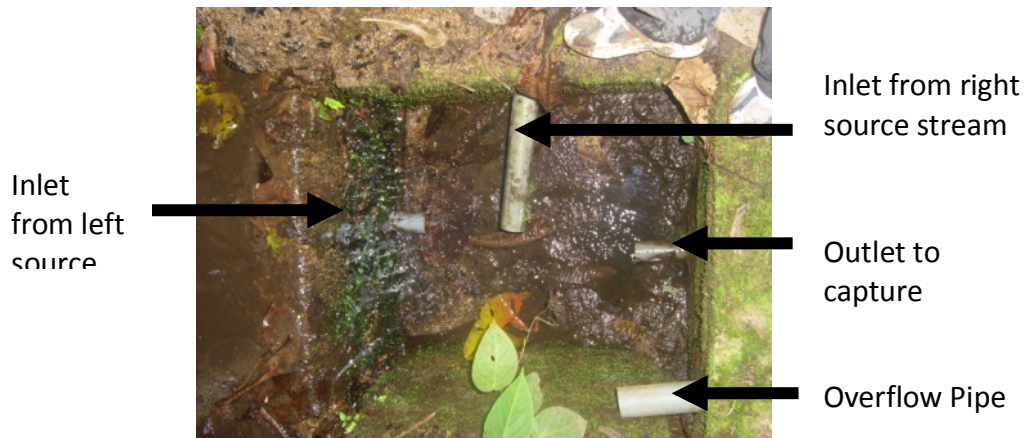
Figure 14: Junction of source streams in the capture box. The travel team noted that before the clogs were removed, the water was only trickling into the box. [55]
