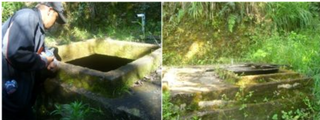
Figure 15: Left and right holding tanks. [55]
