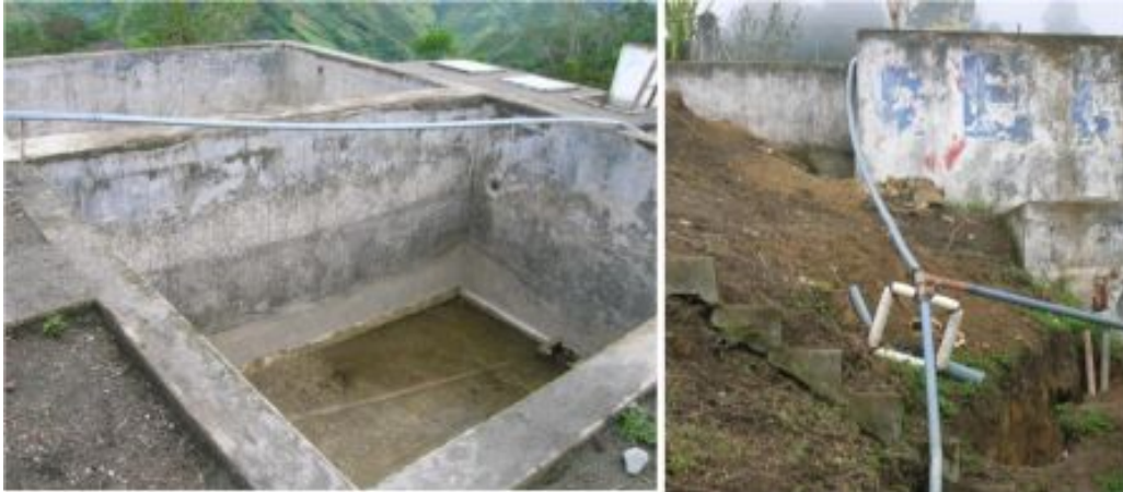
Figure 19: Piped bypass of sand filters 2008 [54]
