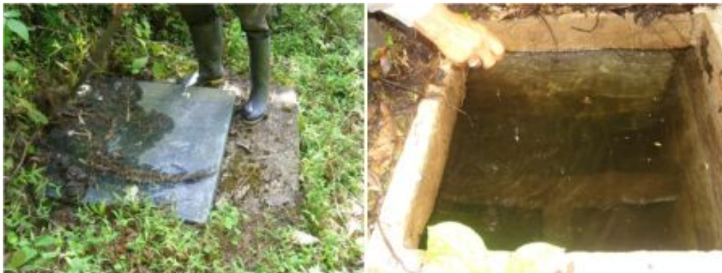
Figure 11: Aeration tanks for El Cristal system. The Tufts EWB travel team noted the presence of animal feces in the left picture. They also noted the generic tank set-up in the right picture, including the T junction to relieve pressure in the piping system. [55]
